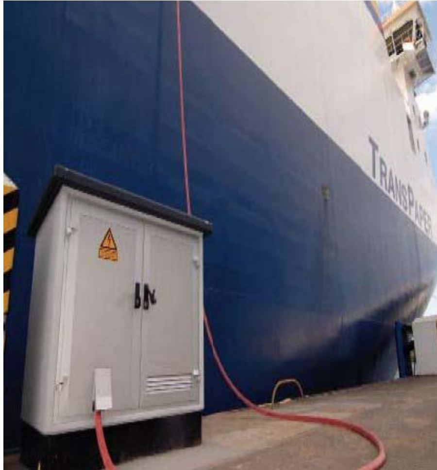
Quelle: Shoreside Power Supply
